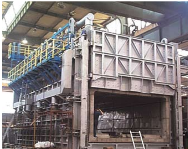
Front view of a conventional-type pusher furnace under shop assembly
