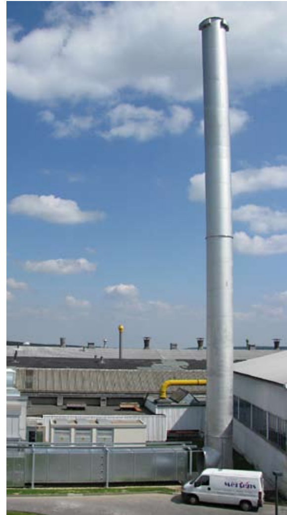
The stainless steel outdoor stack and the heat recovery system
